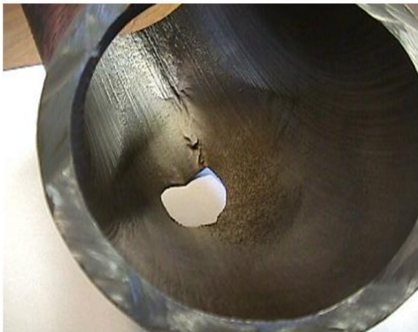
Figure 4-44 – Erosion of a 9Cr-1Mo coker heater return bend.
