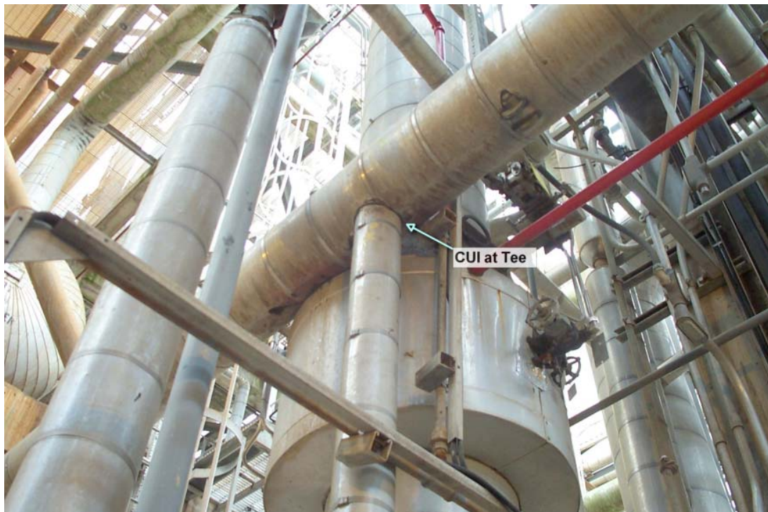
Figure 4-73 – Tee in a 1000 psig ethylene line before insulation removal.
