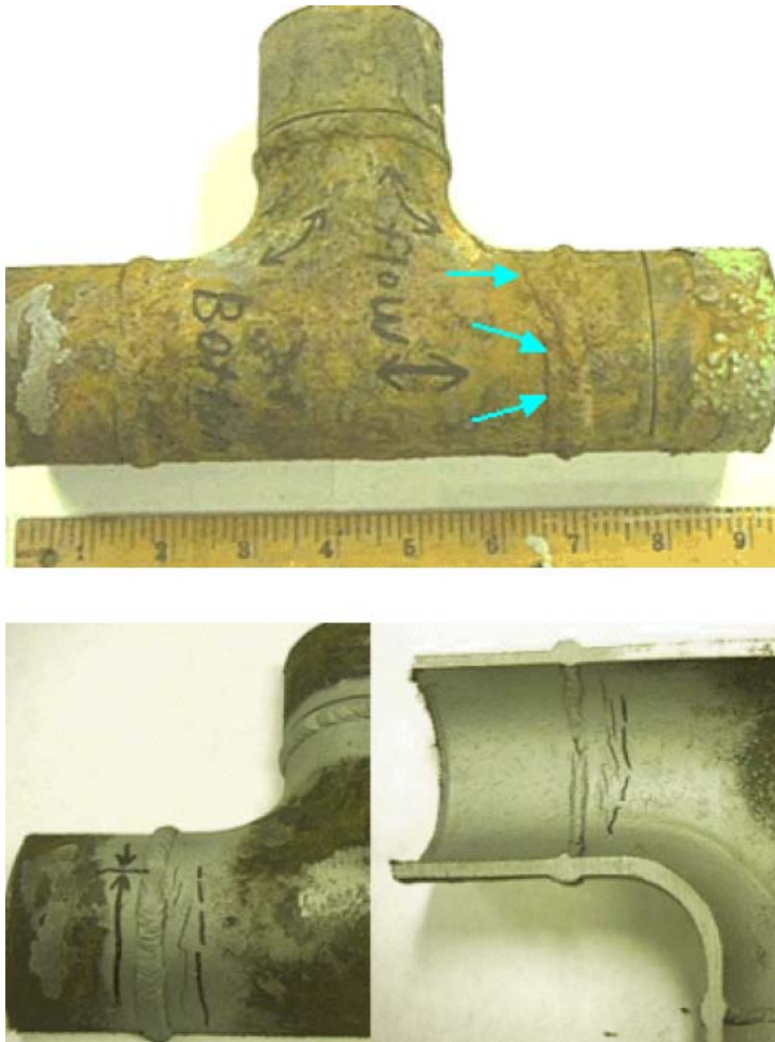
Figure 4-166 – SCC of steel piping in a fuel ethanol system return line/tank transfer line. The top picture shows the crack parallels the pipe-to-tee circumferential weld. The bottom picture shows the inside and outside of the pipe after splitting and cleaning the weld area. Parallel SCC cracks are clearly visible adjacent to the weld.
