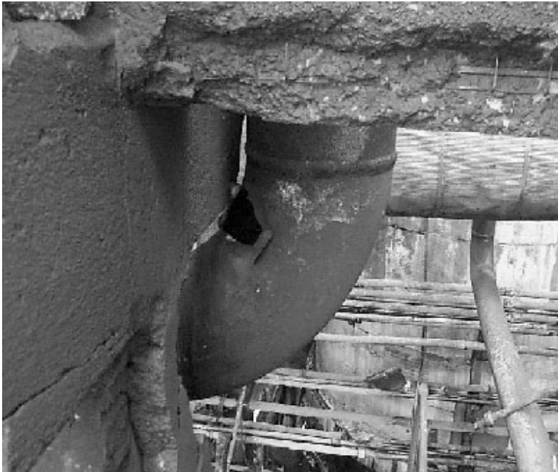
Figure 4-120 – Sulfidation failure of piping elbow.
