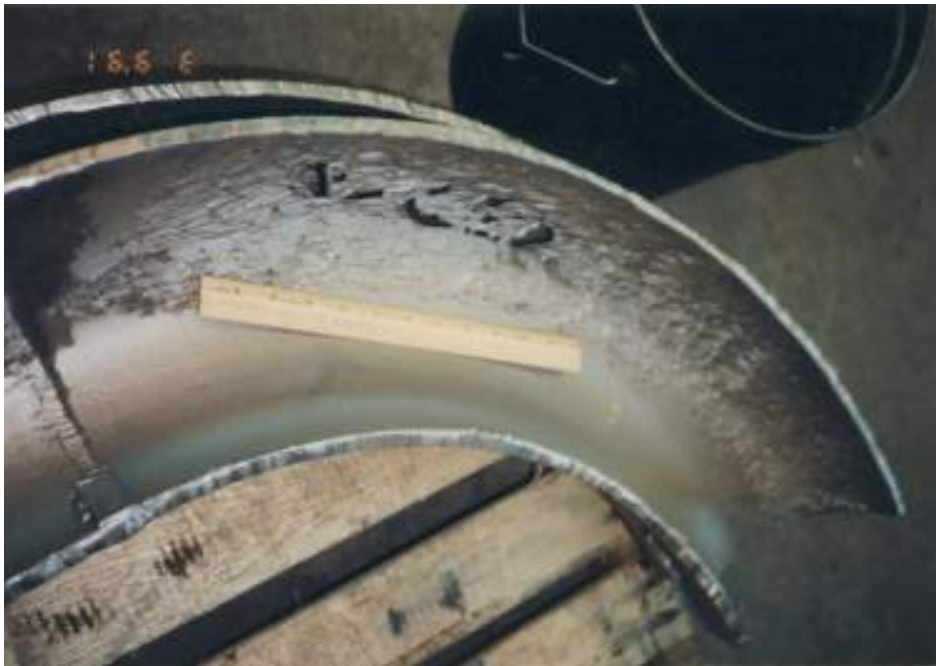
Figure 5-19 – Erosion-corrosion damage due to NAC in a 10-inch 5Cr elbow in the outlet of a vacuum heater in a VDU.
