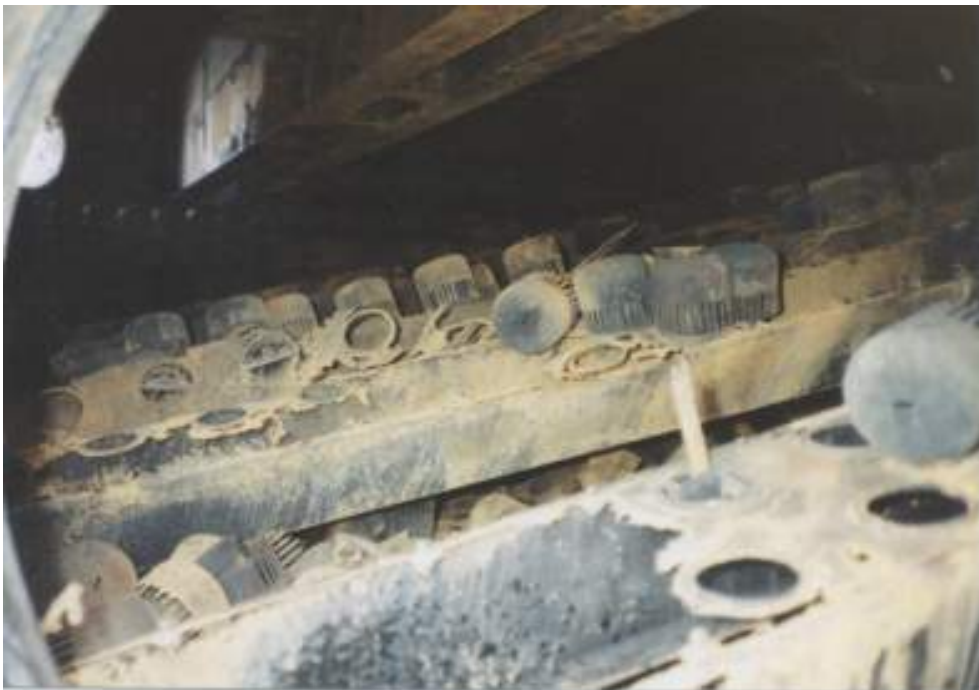
Figure 5-20 – Severe NAC of 410 SS trays and bubble caps in the HVGO section of the vacuum tower fed by the vacuum heater in Figure 5-19.
