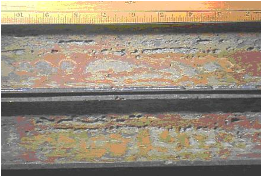
Figure 4-85 – CO 2 corrosion of a carbon steel oil and gas production flow line.
