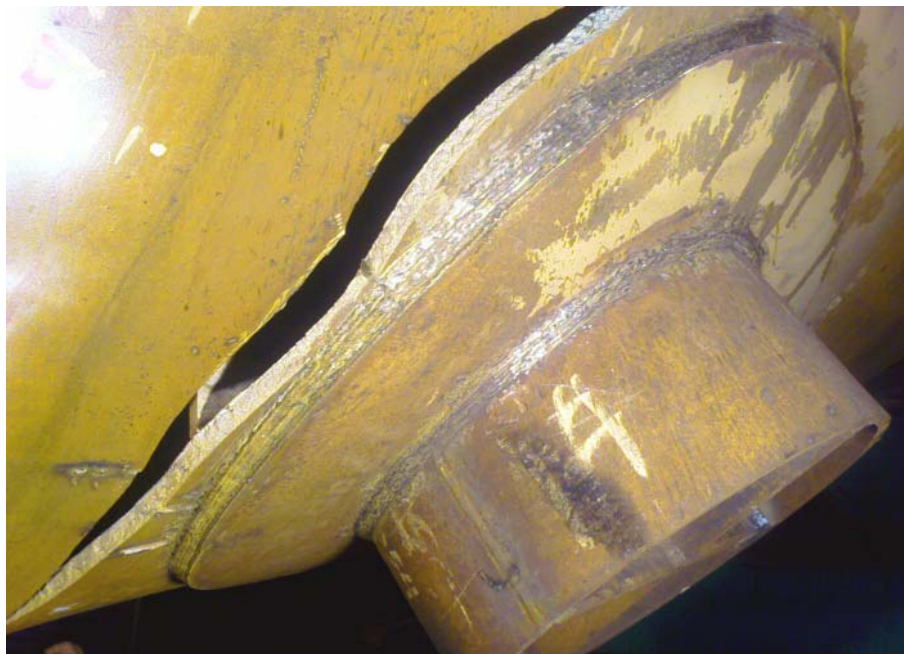
Figure 4-15 – Brittle Fracture of vessel shell during hydrotest.
