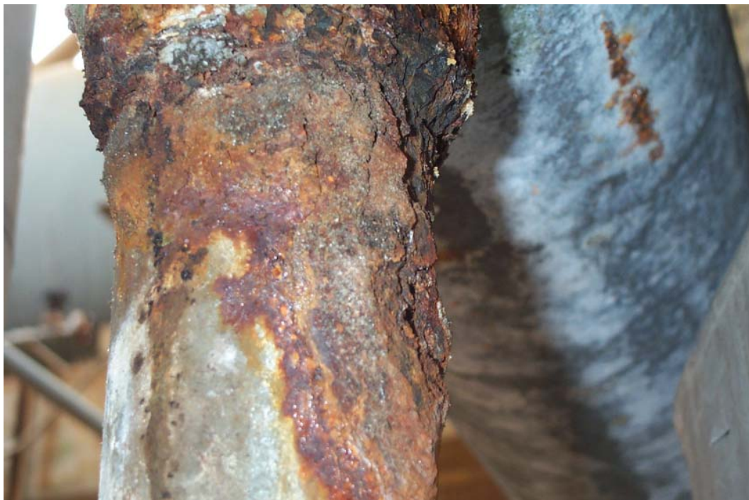
Figure 4-74 – Close-up of Tee CUI of a Tee in Figure 4-73 after insulation removal.
