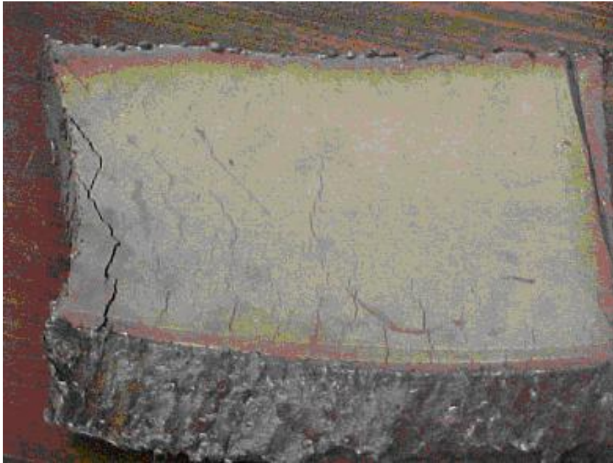
Figure 4-20 – Thermal fatigue cracks on the inside of a heavy wall SS pipe downstream of a cooler H_2 injection into a hot hydrocarbon line.
