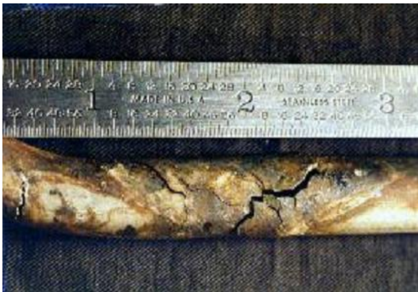
Figure 4-134 – External cracking of Type 304SS instrument tubing under insulation.
