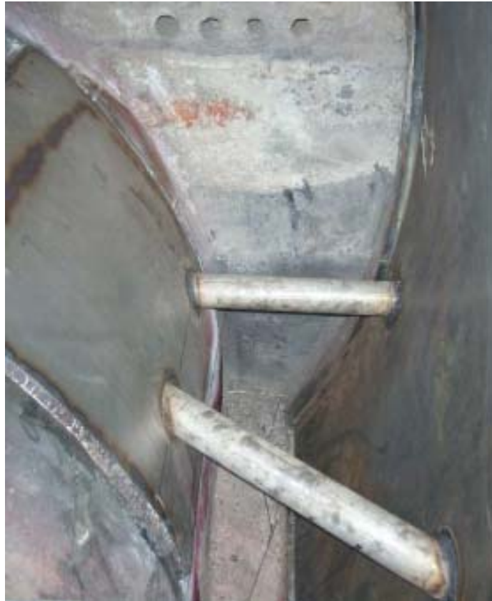
Figure 4-64 – Thermal combustor on the front end of a reaction furnace on a sulfur recovery unit.
