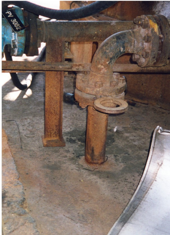
Figure 4-96 – Corrosion of carbon steel pipe at the soil-air interface where the pipe emerges from underground.
