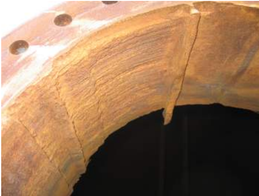
Figure 5-18 – HF Corrosion at manway in HF acid storage service.
