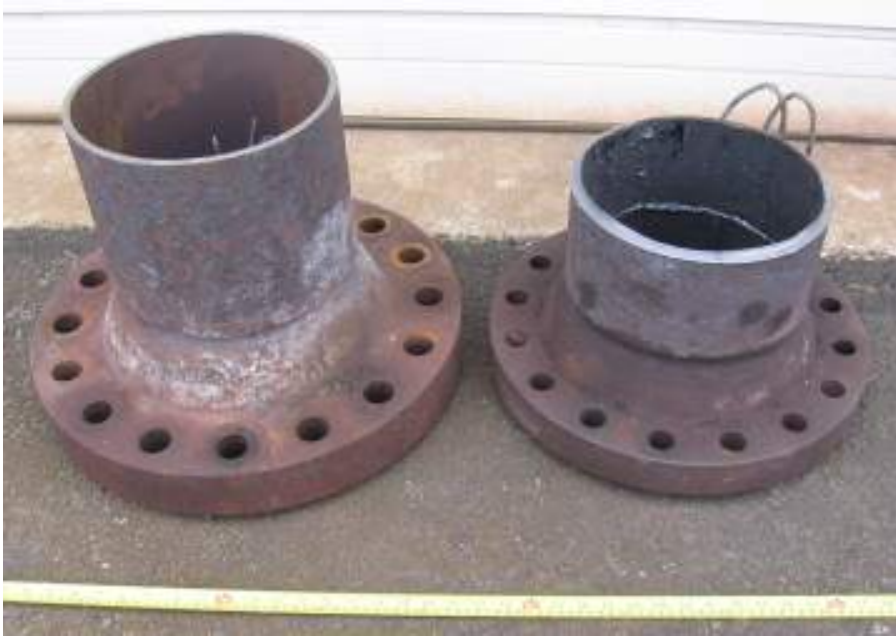
Figure 5-57 – A pair of 10 inch Carbon-0.5Mo flanged pipe sections (SA335-P1 & SA234-WP1) from a hot bypass line in a catalytic reformer that was designed to remain closed but operated partially or fully open for unknown lengths of time. They were in service for ~34 years at temperatures up to 960°F (516°C) and a hydrogen partial pressure of 198 psig (1.37 MPa).
