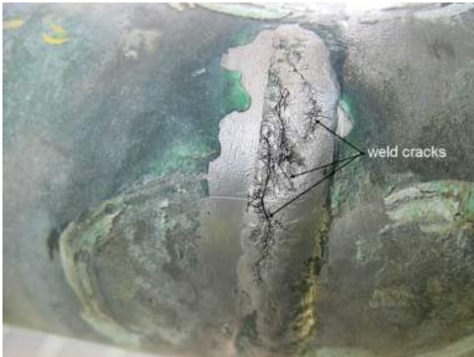
Figure 5-16 – HF stress corrosion cracking of Alloy 400 vent line in an acid dump system (Reference 8).
