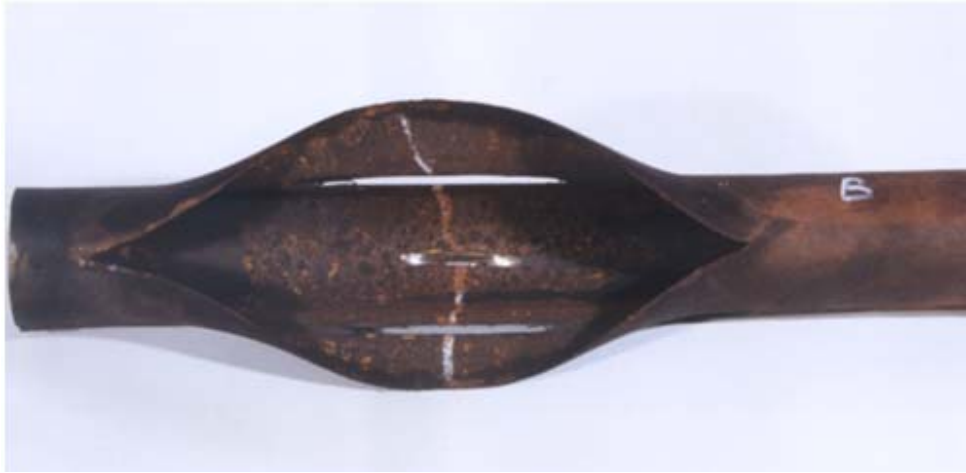
Figure 4-29 – Short term overheating tube failed by bulging and rupture due to short term overheating at a temperature well over 1380°F (750°C).
