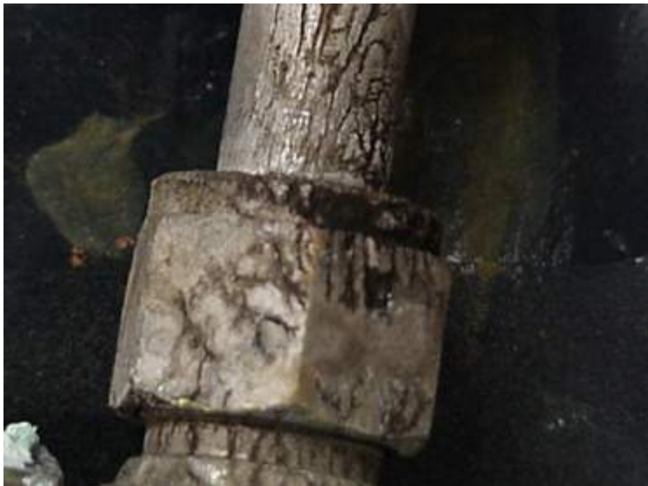
Figure 5-17 – HF stress corrosion cracking of Alloy 400 instrument tubing (Reference 8).
