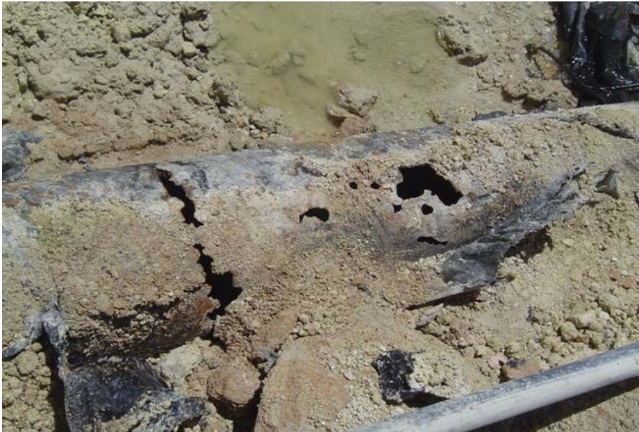
Figure 4-105 – View of the outside of an underground concrete-lined salt water service line that failed from graphitic corrosion.
