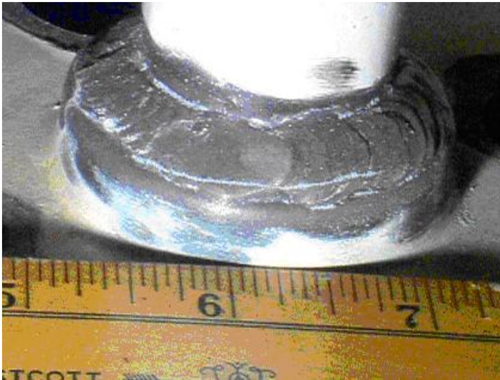
Figure 4-57 – Vibration induced fatigue of a 1-inch socket weld flange in a thermal relief system shortly after startup.
