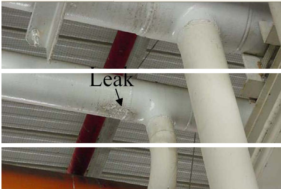
Figure 4-164 – A leak in piping resulting from an ethanol SCC adjacent to the weld.
