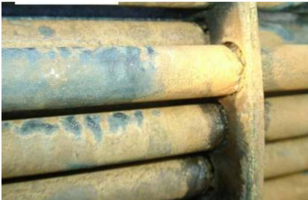
Figure 5-22 – Accelerated corrosion under a baffle.
