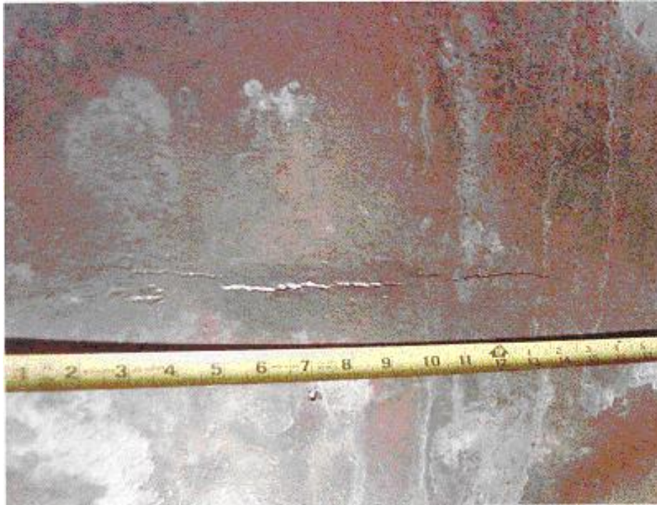
Figure 4-22 –Thermal fatigue cracking associated with bulged skirt shown in Figure 4-21.
