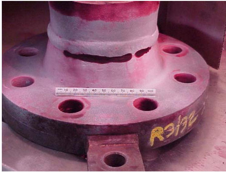
Figure 4-41 – Failure of nickel alloy DMW joining HP40 (Nb modified) tube to 1.25Cr-0.5Mo flange in a Steam Methane Reformer due to cold hydrogen disbonding of the buttering layer. Process temperature 914°-941°F (490° to 505°C), Pressure (2.14 Mpa), H 2 content 10-20% (off-gas).
