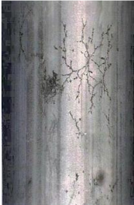
Figure 4-136 – Close-up of the tube in Figure 4-135 showing tight cracks with a spider web appearance.
