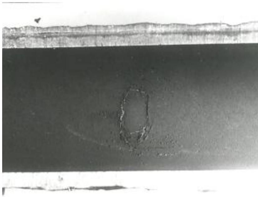
Figure 4-144 – Photograph of a carbon steel boiler tube cut in half lengthwise. Corrosion fatigue cracks initiate at the I.D. of a tube, opposite a buckstay attachment on the O.D. (Mag. 1X)
