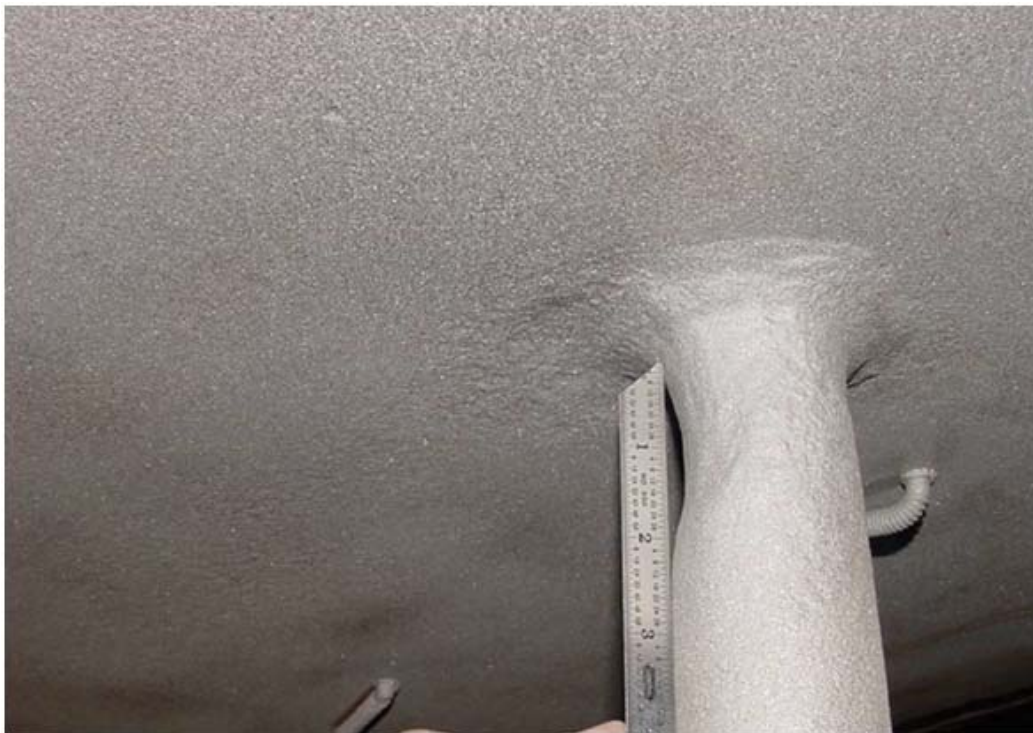
Figure 4-76 – CUI of nozzle on a bottom head.
