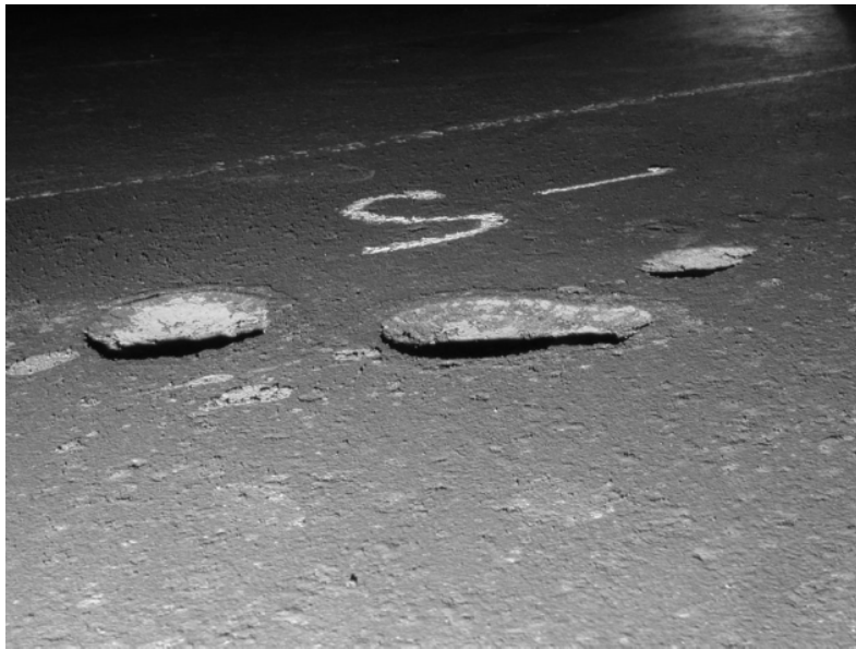
Figure 4-89 – MIC of diesel tank bottom.
