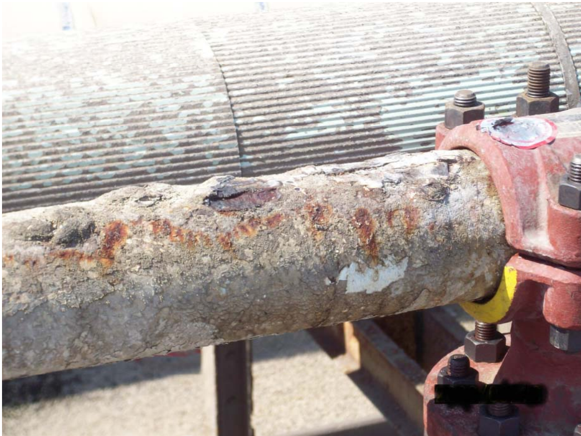
Figure 4-72 – Atmospheric Corrosion of an LPG line in close proximity to a cooling tower.
