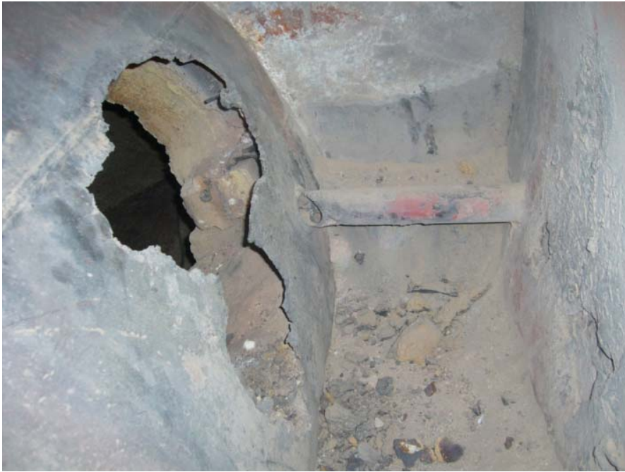
Figure 4-65 – Same as figure above after damage due to oxygen combustion resulting from oxygen injection into the thermal combustor on the front end of the reaction furnace.
