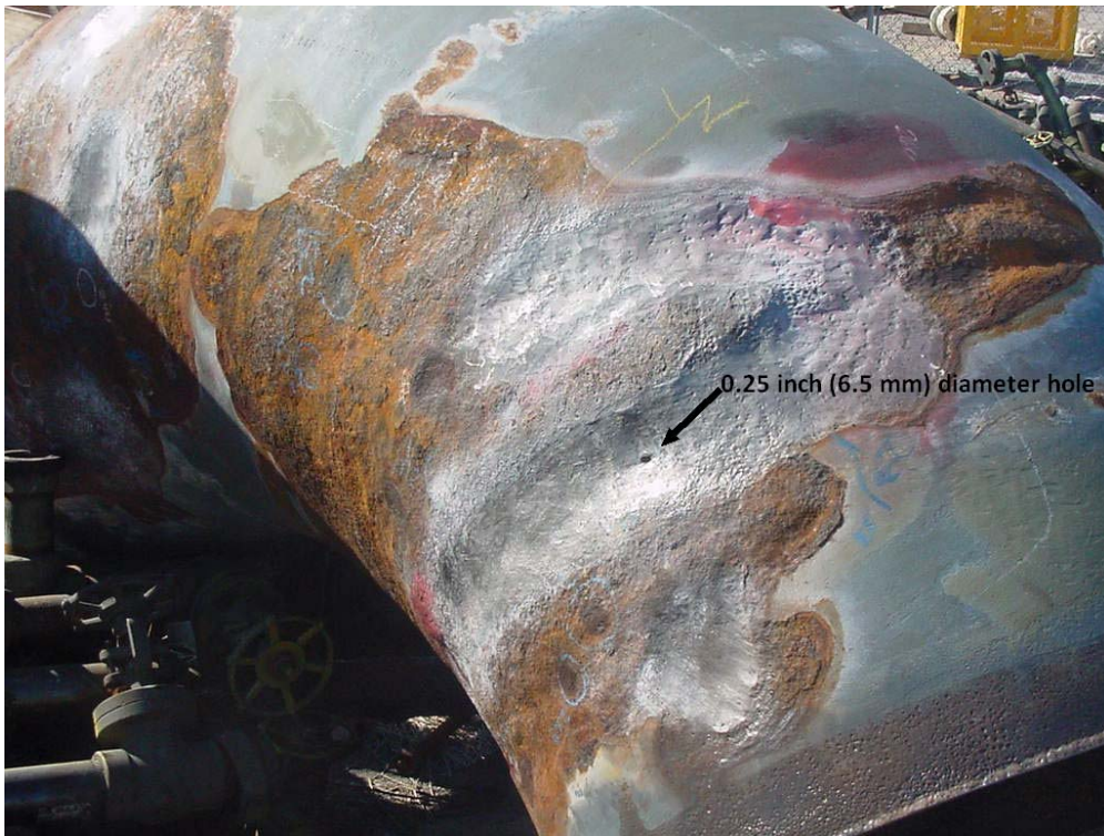
Figure 4-75 – CUI of a 30 inch CS Butadiene line showing highly localized corrosion which could only be found by stripping the entire line. Note the 0.25 in (6.5 mm) diameter hole at arrow.
