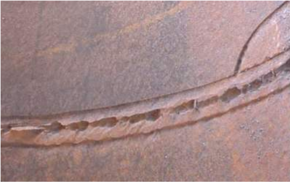
Figure 5-3 – Preferential weld corrosion in lean amine (Reference 5)
