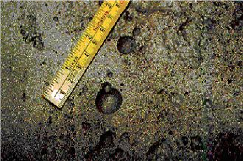
Figure 4-93 – Same oil line as Figure 4-92. Hemispherical pitting typical of MIC can be seen after grit blasting to remove the scale.
